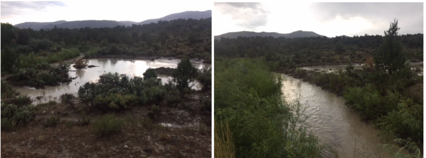
Photo 5 and Photo 6: Flooding at confluence of unnamed drainage and Stewart Ditch and sediment deposition above the ditch plugging the culvert. Photo Credit Elaine Brett.
