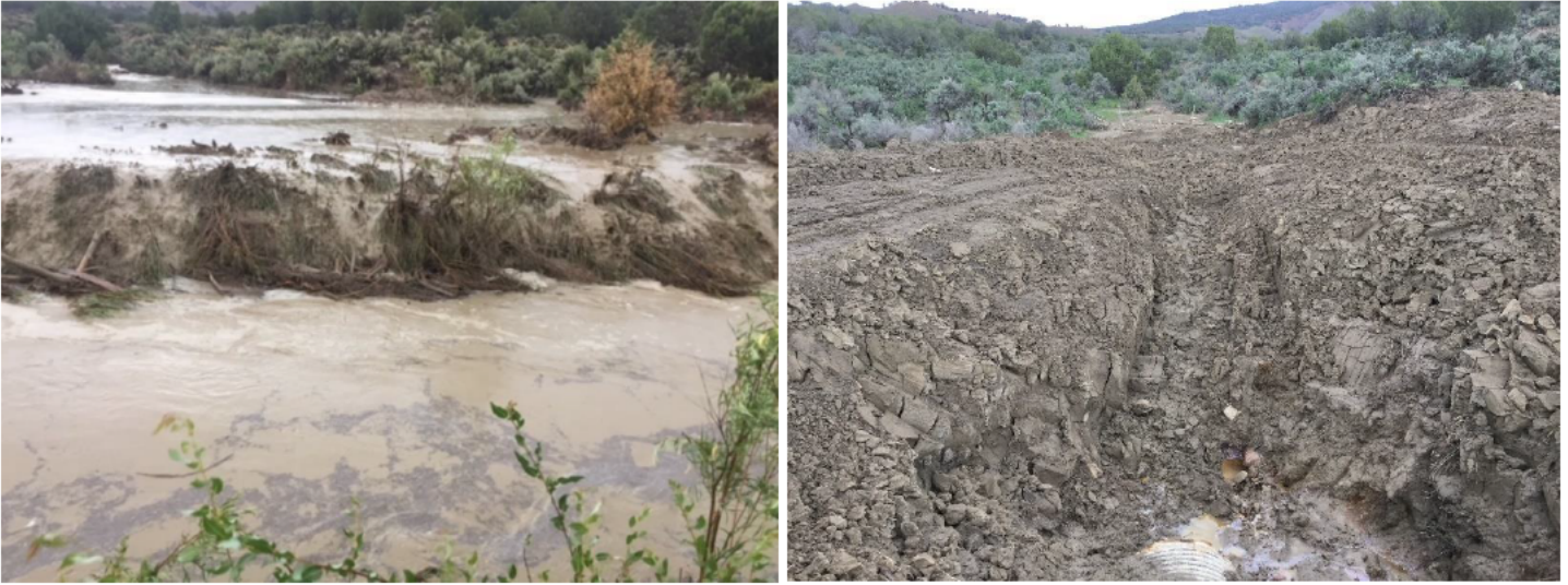
Photo 7 and Photo 8: Flooding at confluence of unnamed drainage and Stewart Ditch and sediment deposition above the ditch plugging the culvert. Photo Credit Elaine Brett.
