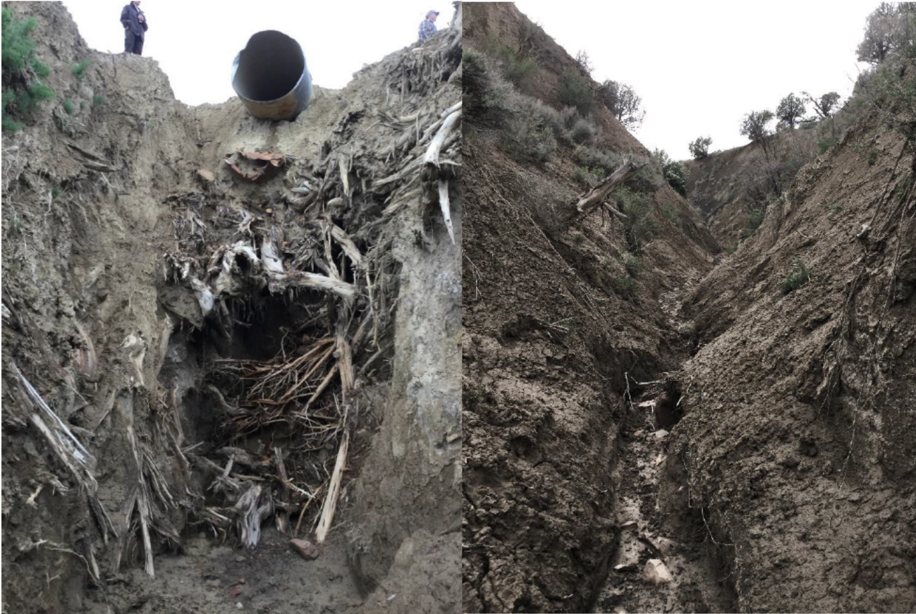
Photo 3 Photo 4 Western Area Power Authority (WAPA) road crossing at an unnamed natural drainage.
